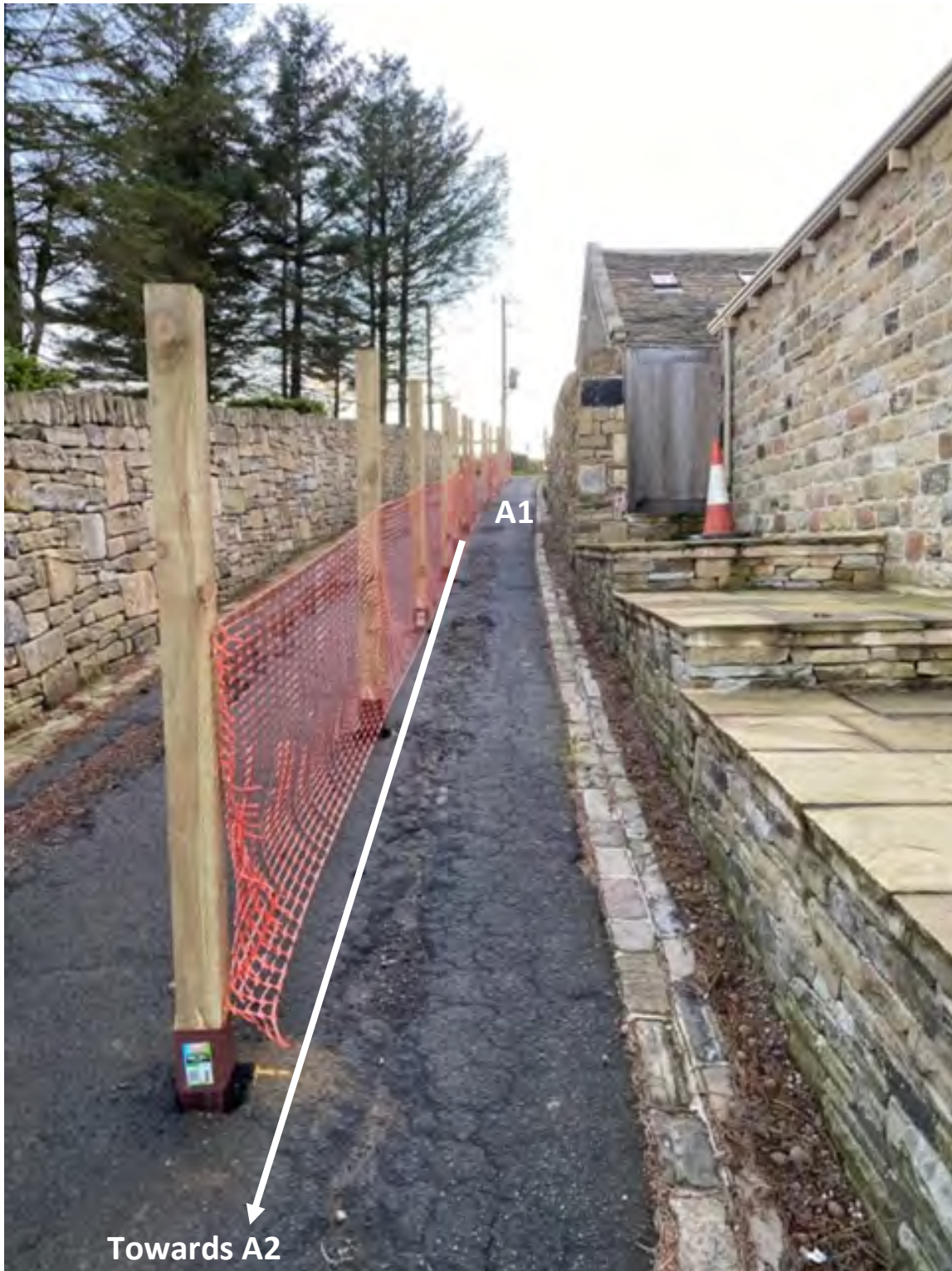
19. View west towards point A1 from near A2 showing line of fence posts erected in early September narrowing the usable width of the driveway (path Holmfirth 60) to approx. 1.2m. 21 Oct 2020.
