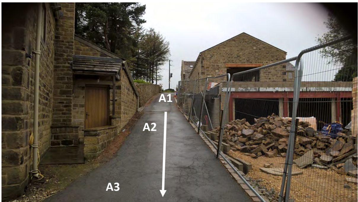
16. View east from the corner of the house at A3, looking west up the driveway toward point A point A. Similar position to above at A1 looking towards point A. The fire damaged outshut at A2 had been rebuilt. Work was underway to construct a new garage block on the north side of the driveway. 11 Jun 2019.
